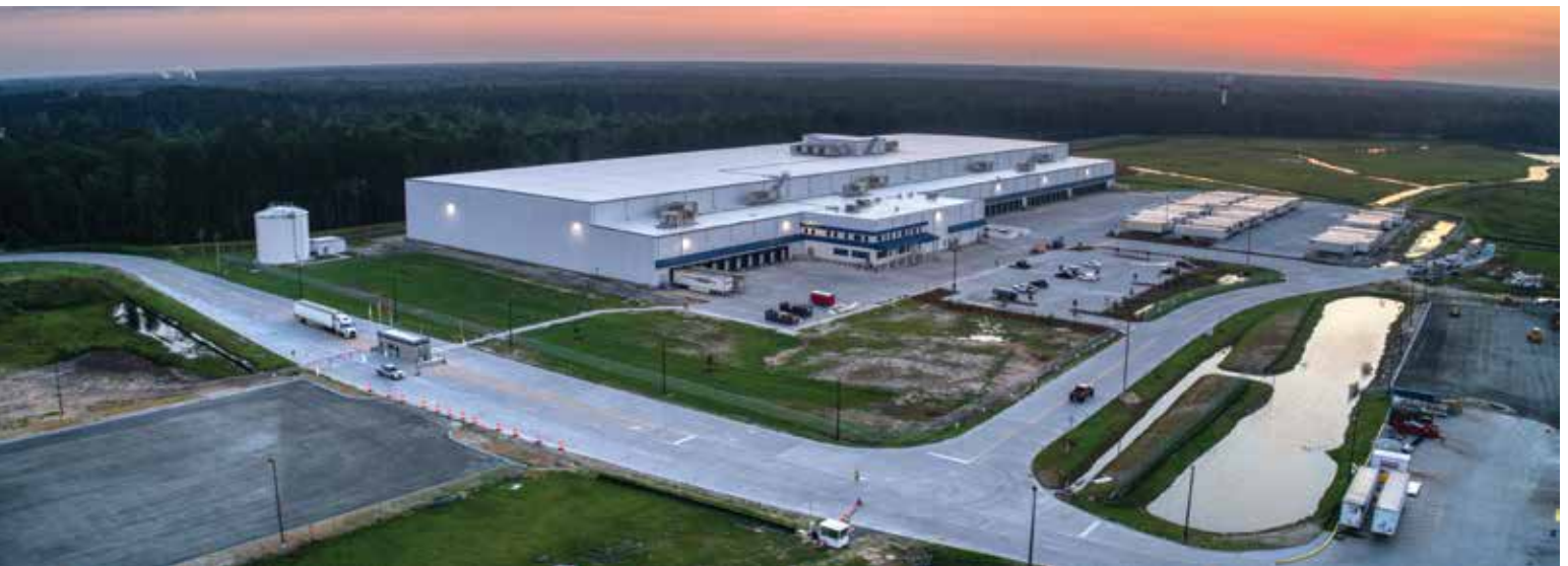
Because of the area's high groundwater, gravel was laid and water continuously pumped offsite to stabilize the ground for construction activities. (Photo courtesy of Primus Builders.)
