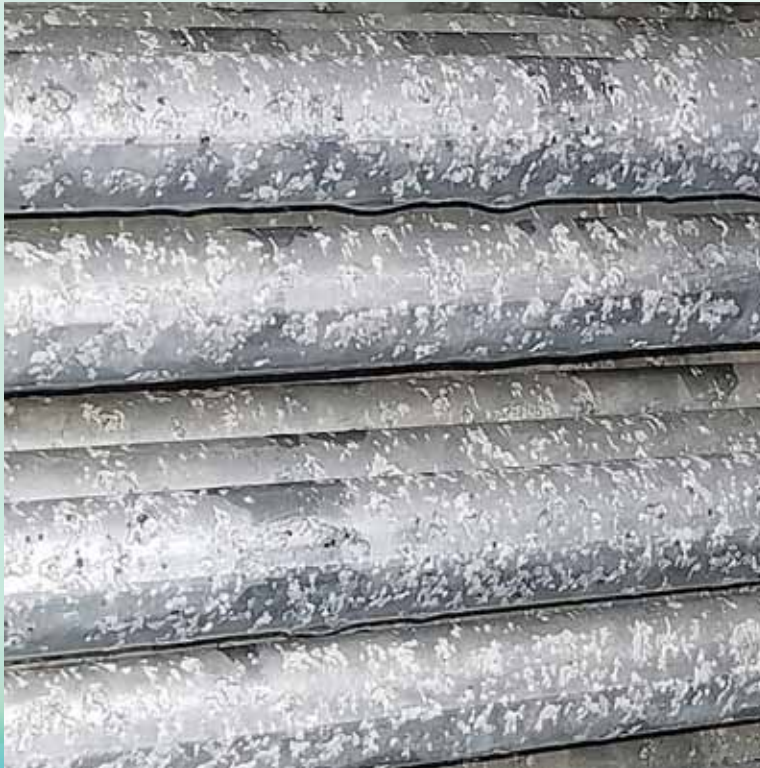
White Rusted Coil without Pass-Protect
