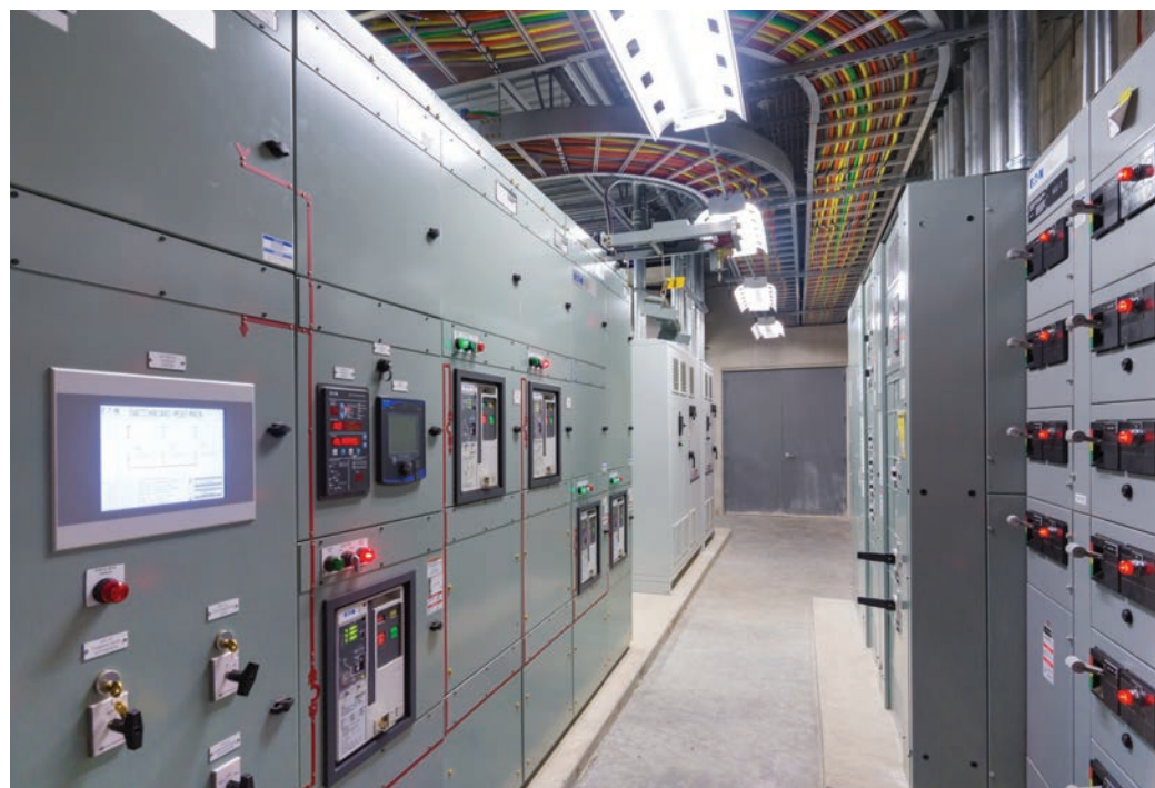
The new electrical room at Bahamas Food Services includes a switchgear lineup in front and large compressor VFDs in the rear (right side) MCC sections on the left (more motors).
