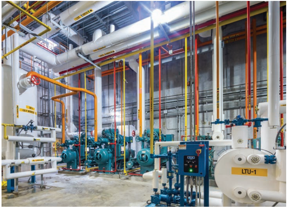
The machine room that Stellar designed at Bahamas Food Services refrigerated distribution center includes a liquid transfer unit and +35 degree intercooler vessel.
