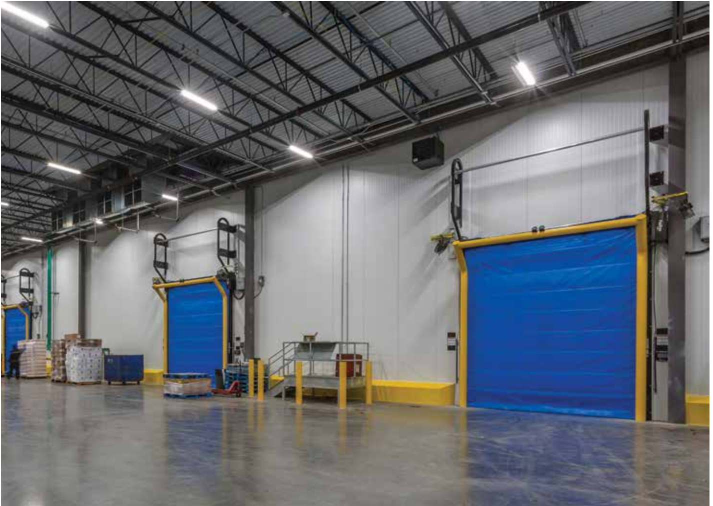
Recycled, crushed, and reused demolished concrete served as an under-slab granular fill base for cooler, freezer and cold dock slabs on grade. (Photo courtesy of Williams Company.)
