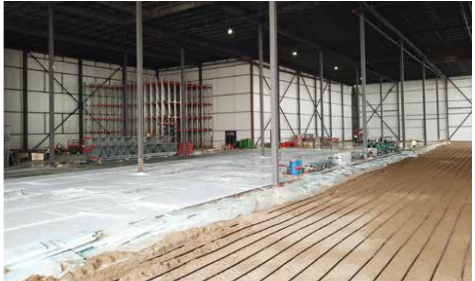
In the background, progress is shown of an expedited zone that was needed while floors were still being established (in the foreground) and racking installed. (Photo courtesy of Coldbox.)
