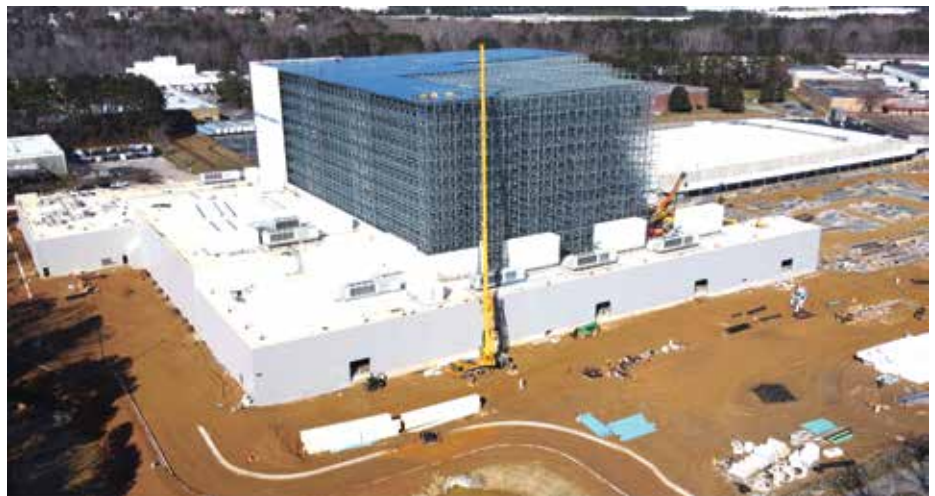
The 150-foot, -10-degree ASRS, included 41,000 pallet positions. (Photo courtesy of Griffco Design/Build.)
