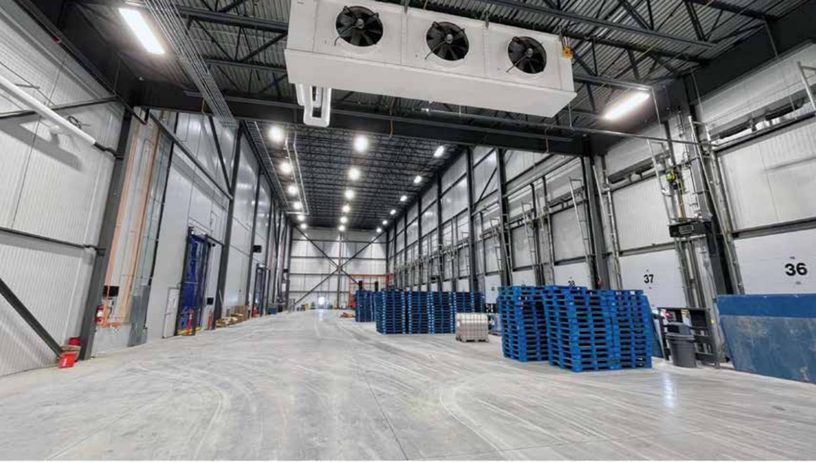
The cold dock floor system included insulation that increased the R-value, reducing the refrigeration load. (Photo courtesy of Coldbox.)
