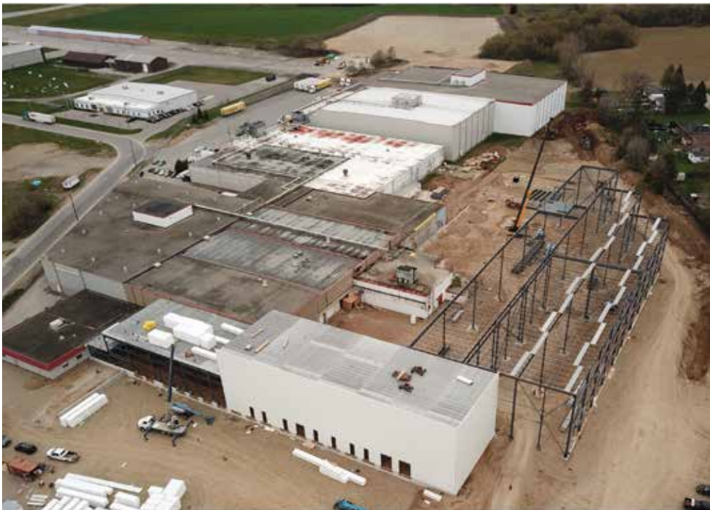
The existing facility with the new facility construction underway. The engine room is isolated (in the middle of the photo) following demolition. (Photo courtesy of Coldbox.)
