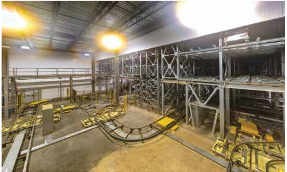
The subsystems were connected by an Electrified Floor Track System by Eisenmann, which moves product between locations and then to the shipping dock. (Photo courtesy of Griffco Design/Build.)
