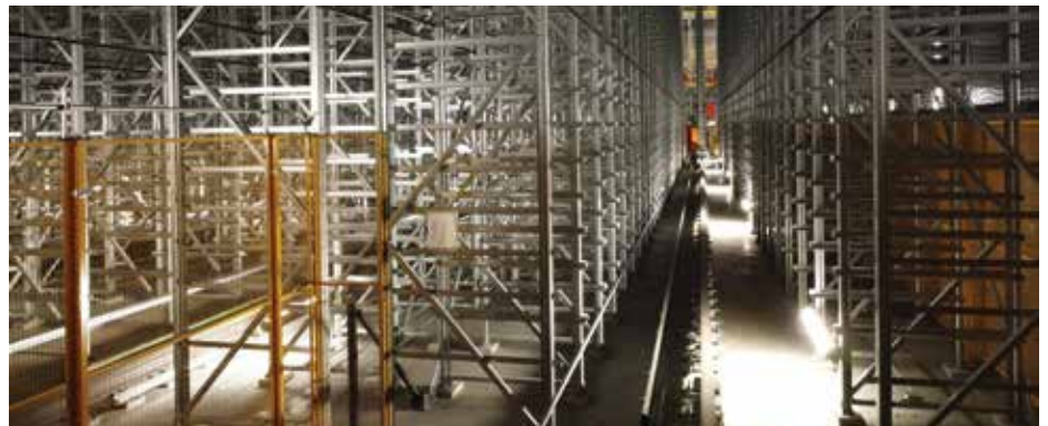
Because of the low oxygen nature of the freezer, all pallets in and out of the freezer are handled by an automation system comprised of conveyors, monorails and cranes. (Photo courtesy of Fisher Construction Group.)
