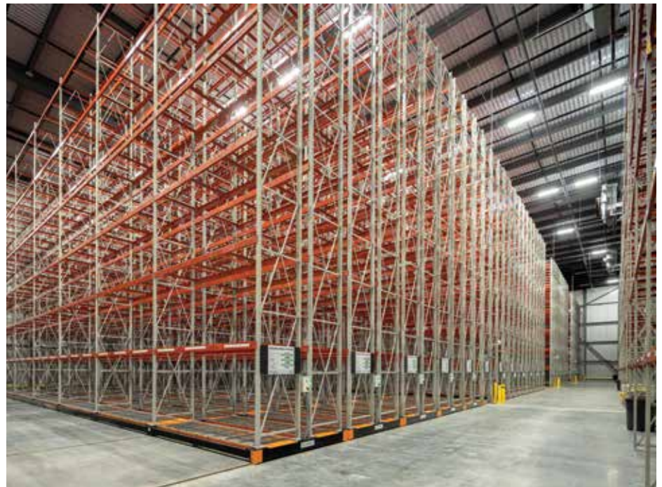
Flex space mobile racking in the finished facility. (Photo courtesy of Ti Cold.)
