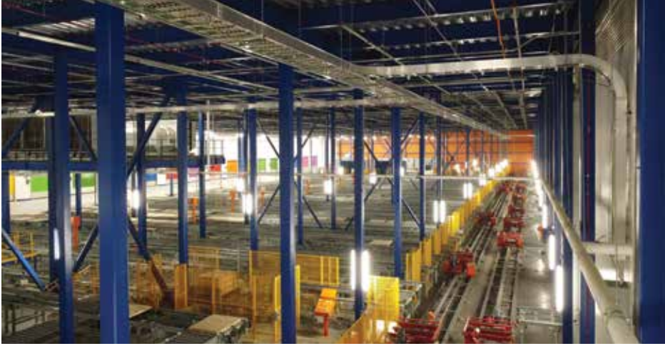
Once a pallet is unloaded, it is placed on an inbound conveyor where the system tracks each pallet and designates it a position in the freezer. (Photo courtesy of Fisher Construction Group.)
