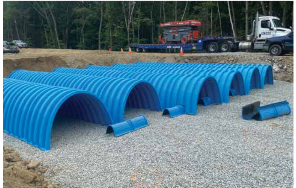
Underground storm drainage basins were used because of the tight site space. (Photo courtesy of Ti Cold.)
