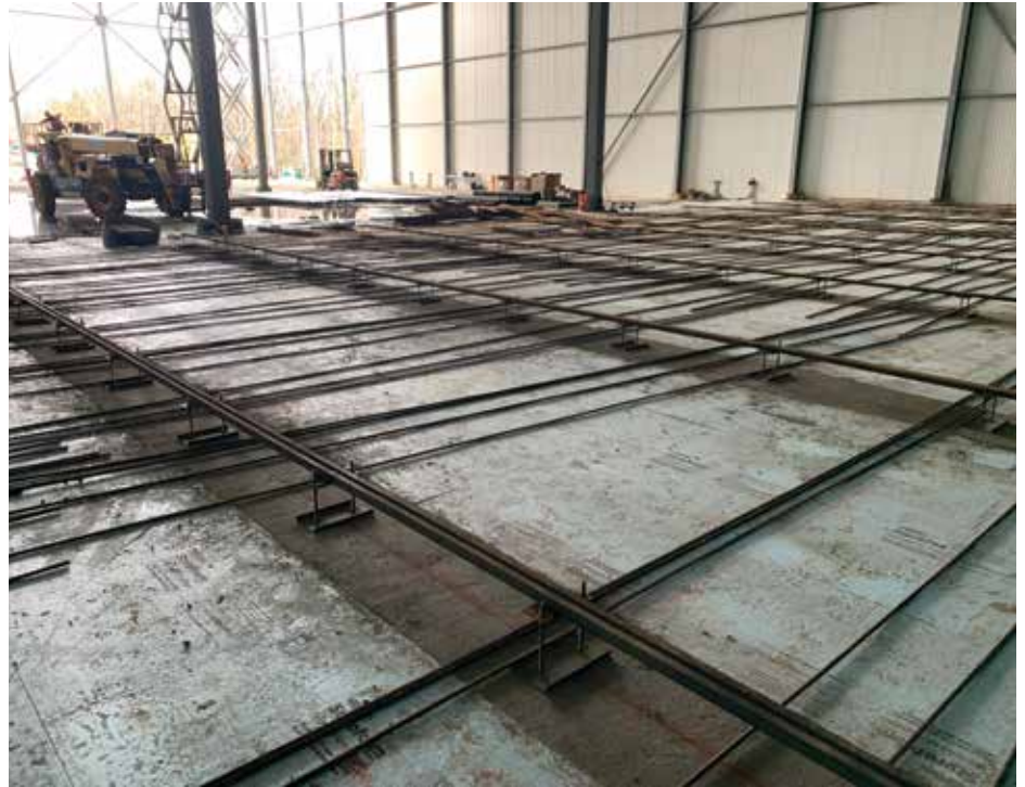
The racking rails, seen here pre-pour, had to be precision calibrated. (Photo courtesy of Ti Cold.)
