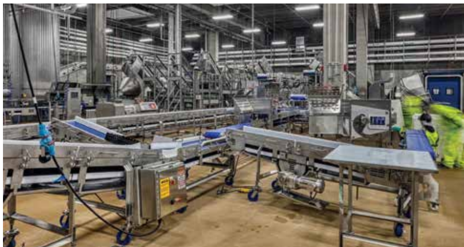
Big-D Construction built a modern processing facility for Riverbend Ranch with the capability to humanely process animals from harvest to finished packaged product. (Photo courtesy of Big-D Construction.)
