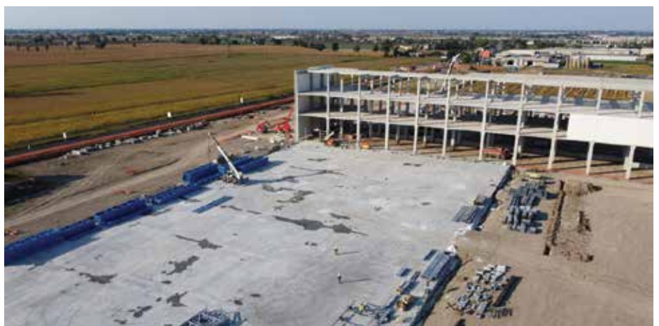
Illustrating the progress that has been made since the early stages of the build. (Photo by Flavio Chiesa courtesy of NewCold.)
