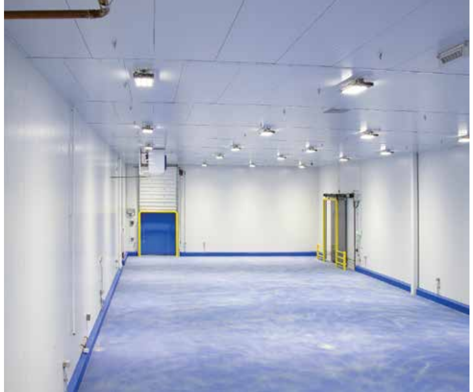
Ceiling-only sprinkler systems, which do not require in-rack sprinklers, are currently capable of providing protection up to 55 feet. (Photo courtesy of Fisher Construction.)
