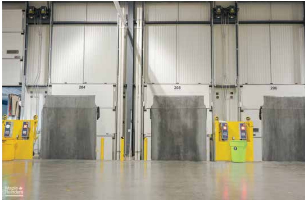
The build features a 30,000 square foot cooler/cold dock with levelers. (Photo courtesy of Maple Reinders.)
