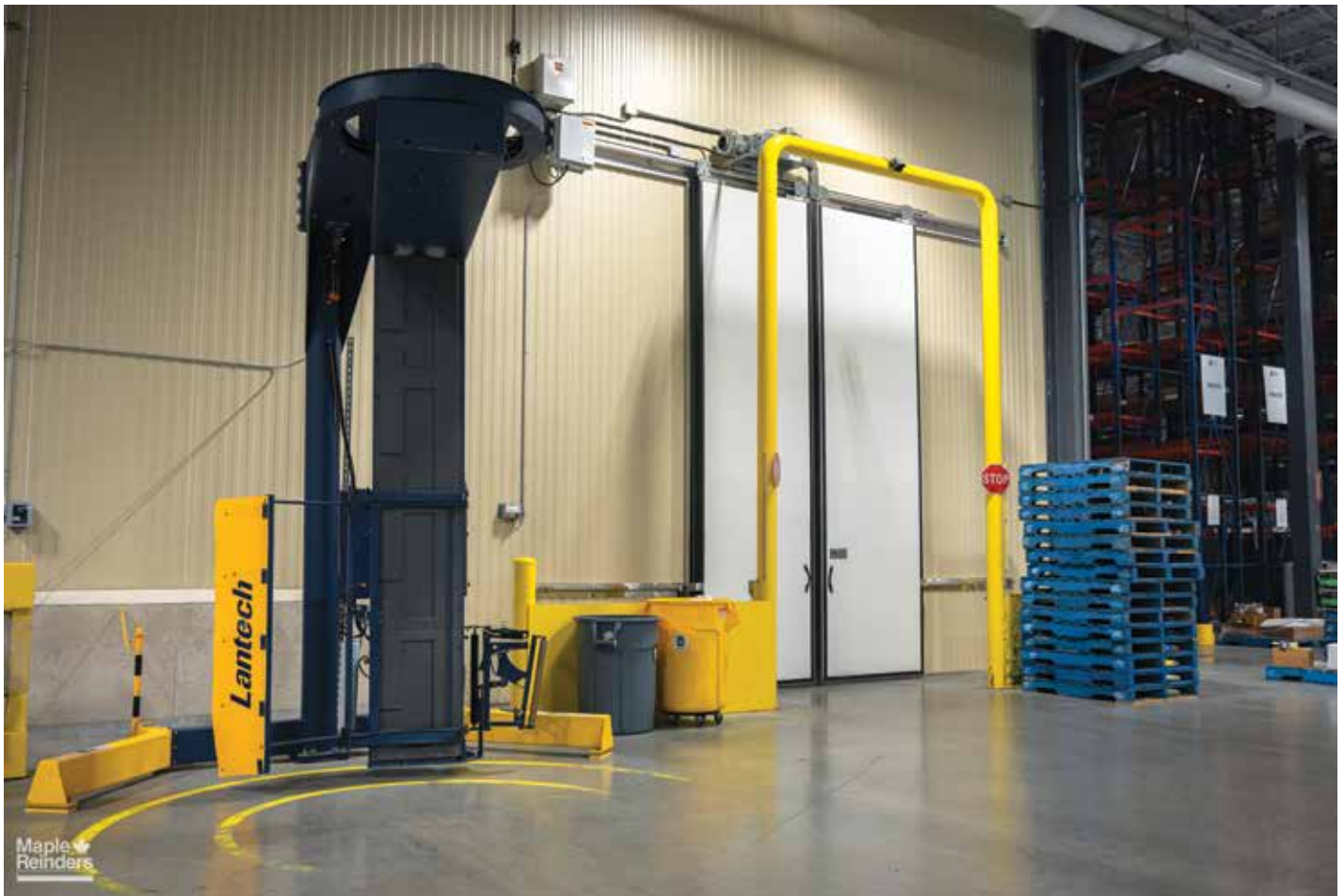
A pallet wrapper with roll-up door in the background at Dot Foods’ new distribution center. (Photo courtesy of Maple Reinders.)
