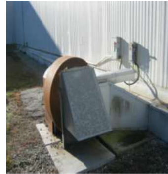
Figure 5.6 Forced Air Unit
