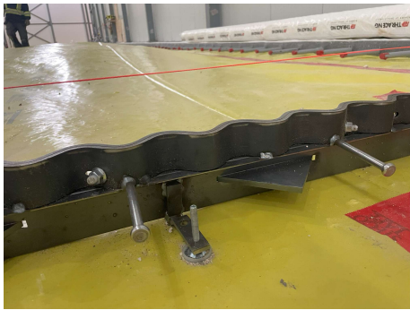
A sinusoidal, dowelled, concrete armor joint system being installed over a radon barrier in a food service facility. Courtesy Alphacon, Inc.
