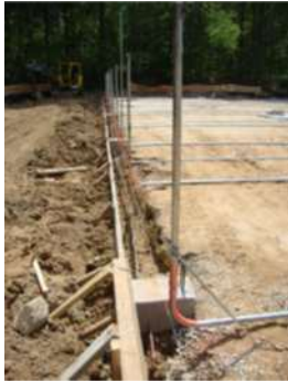
Figure 5.7 Electrical heat conduit
