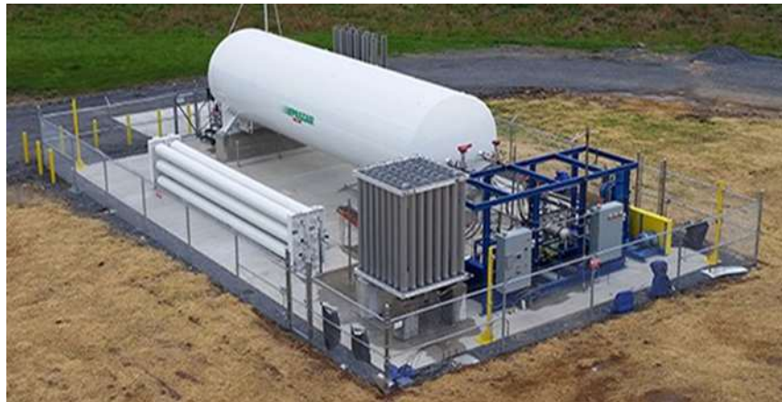
Figure 11.19 Outside Hydrogen Generator and Storage Unit
