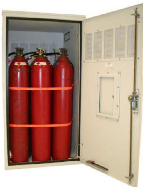
Figure 11. 18 Hydrogen Storage Cabinet
