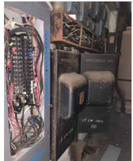
Above: Interior cooling system. Below: An old electrical panel. (Photos courtesy of Americold.)
